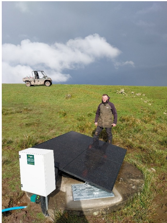
Solar powered pump for livestock watering funded by a Farming in Protected Landscapes grant
